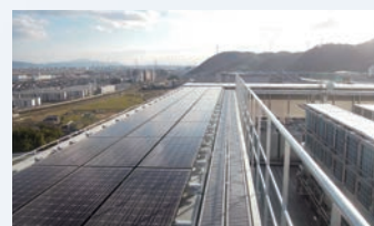
Solar panels (Minase Research Institute)
