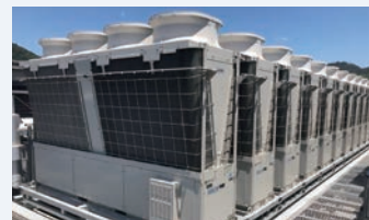
Module-type heat pump chillers (Minase Research Institute)
