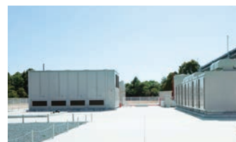
Large-capacity electricity storage system (Yamaguchi Plant)
